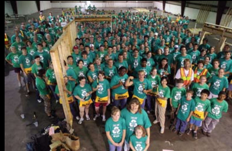
Behavioral science volunteers, along with others from the Drury family, work on Springfield's first sustainable house for Habitat for Humanity.
